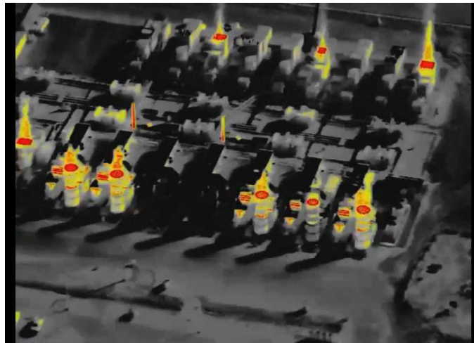
Figure 2. Thermal camera image of xAI's Stanton Road S. facility (Oct. 31, 2025; Steve Jones/SouthWings).
