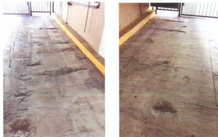
Figure J2: Spalling with exposed steel reinforcement at topside of garage deck.
