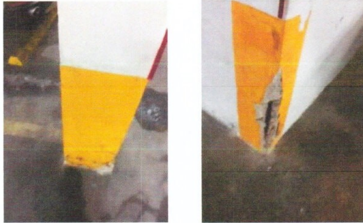
Figure J1: Typical cracking and spalling at parking garage columns
