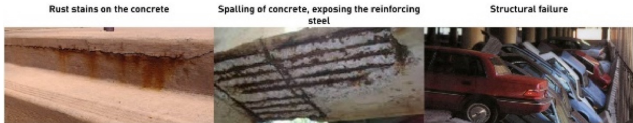
Stages of visible deterioration.
