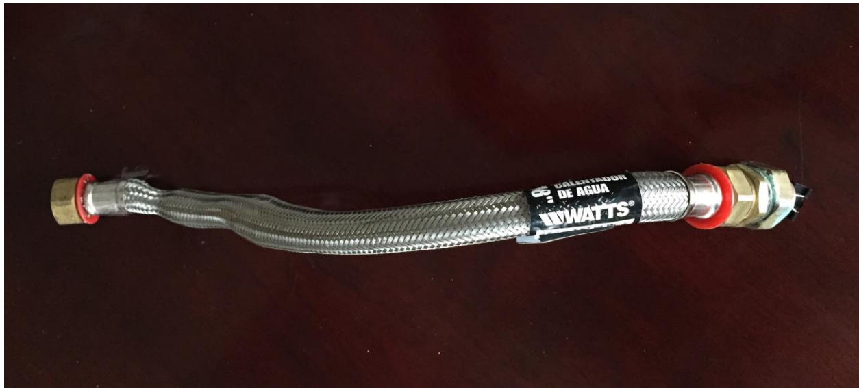
Figure 1 : Full View of Failed Line
