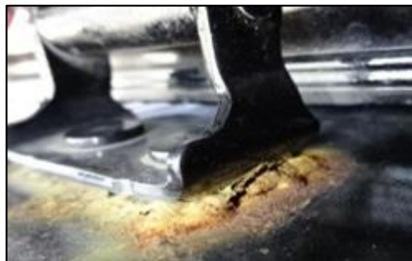
Figure 2. Defined Red Rust
