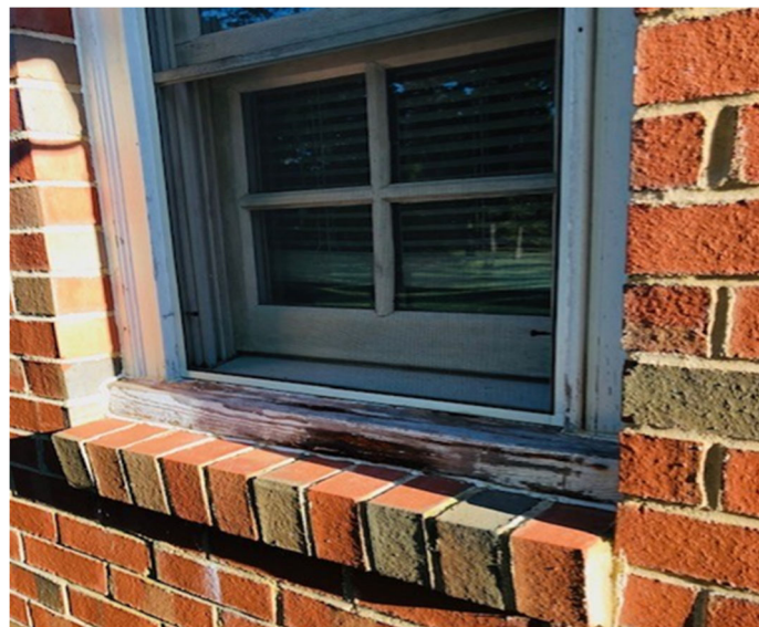
Photograph 32: Rotting Window Sill
