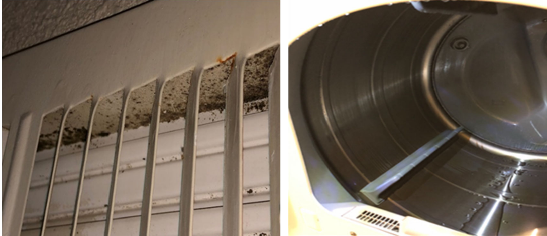
Photographs 39 and 40: Rust, Mold, and Condensation
