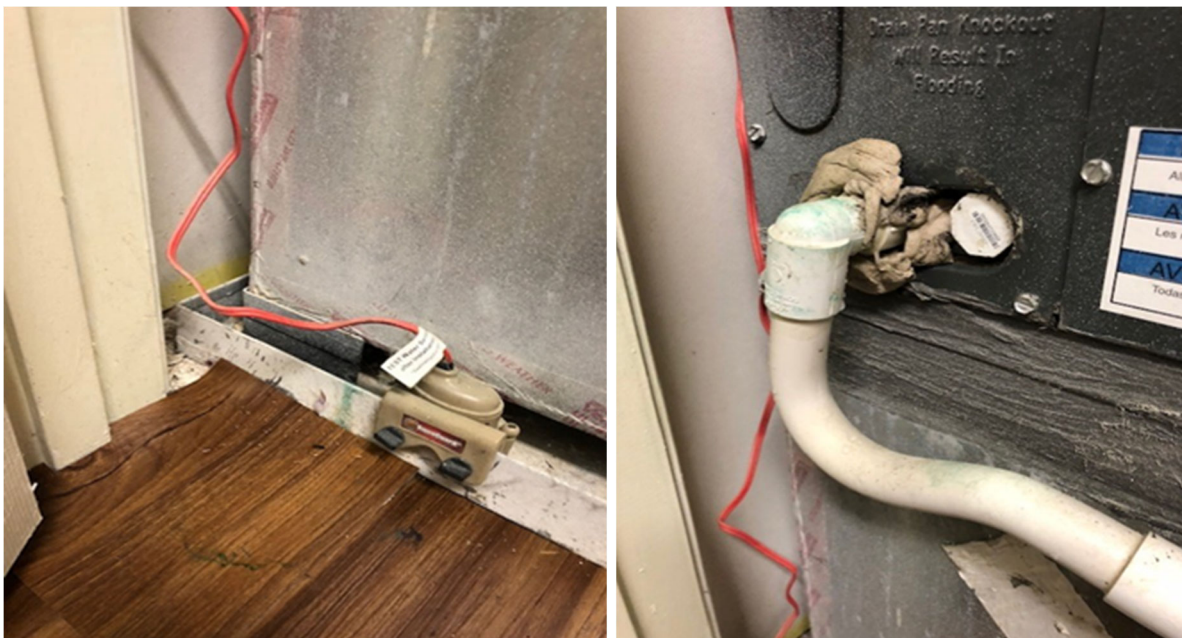
Photographs 20 and 21: Water Damage from Leak and Putty Wrapped around Pipe
