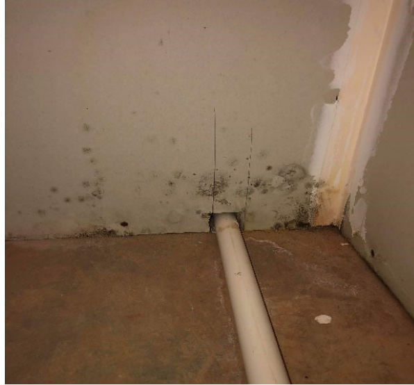
Photograph 5: Fungal Growth in Storage Closet
