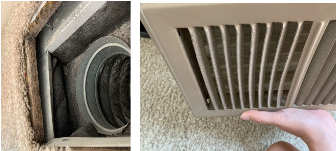
Photographs 3 and 4: Mold on Subfloor and Vent
