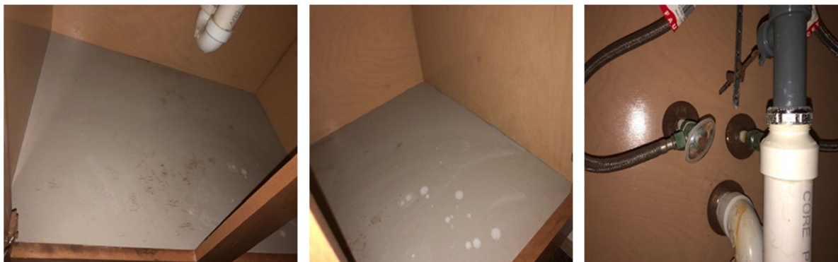
Photographs 34, 35, and 36: Water Damage Under Cabinet
