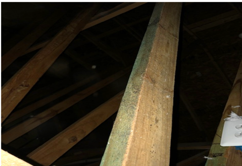
Photograph 33: Mold in Attic
