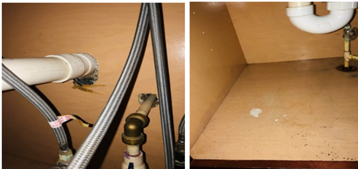
Photographs 18 and 19: Water Staining Under Sink
