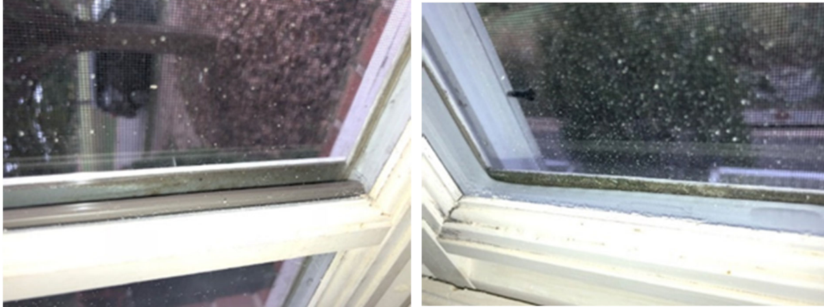
Photographs 29 and 30: Mold in Windows
