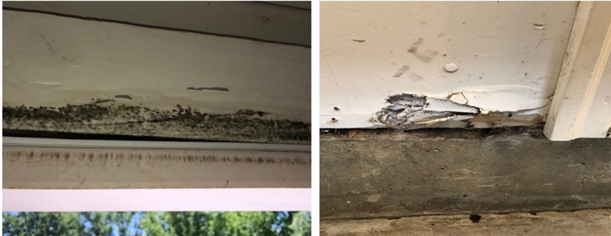
Photographs 10 and 11: Mold and Evidence of Water Intrusion
