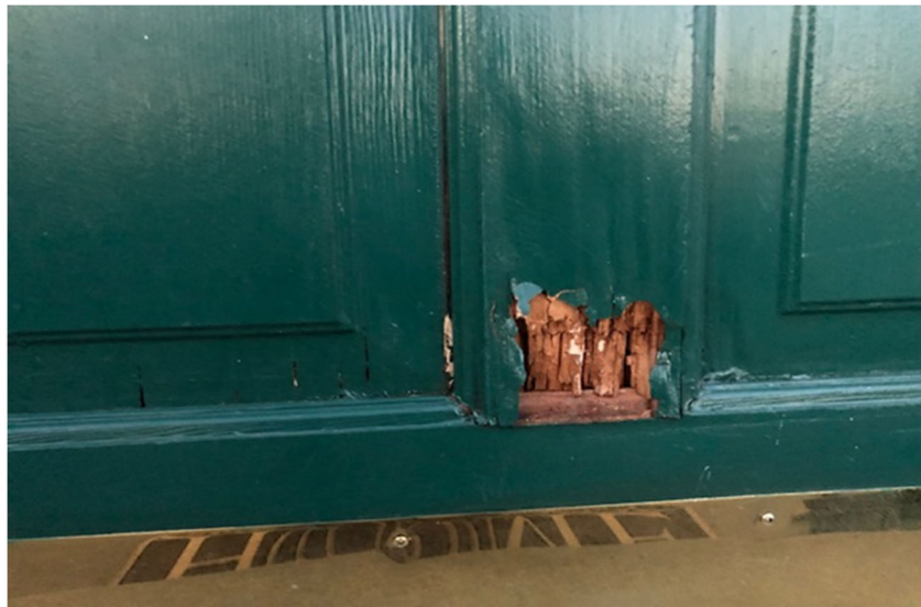
Photograph 31: Rotting Wood Door
