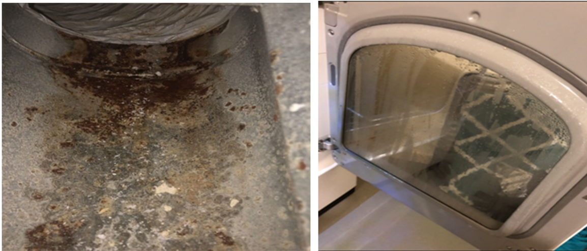
Photographs 41 and 42: Rust, Mold, and Condensation
