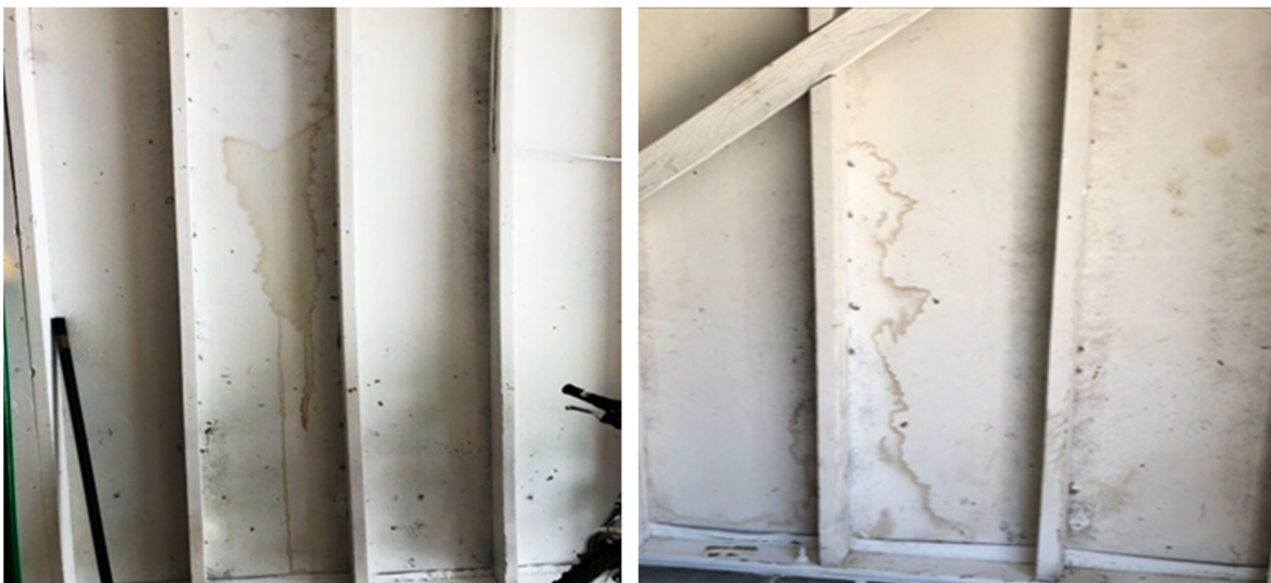
Photographs 16 and 17: Water Damage
