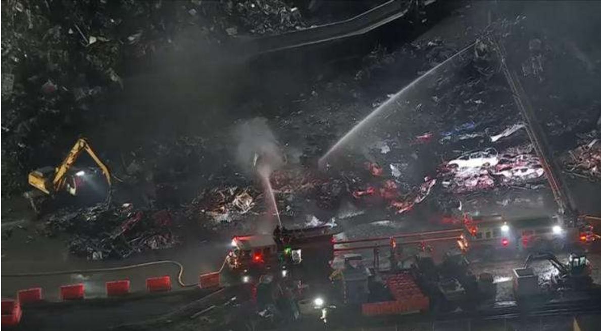
[Overhead view of February 26, 2026 fire at Defendant EMR Metal Recycling, LLC's Facility]
