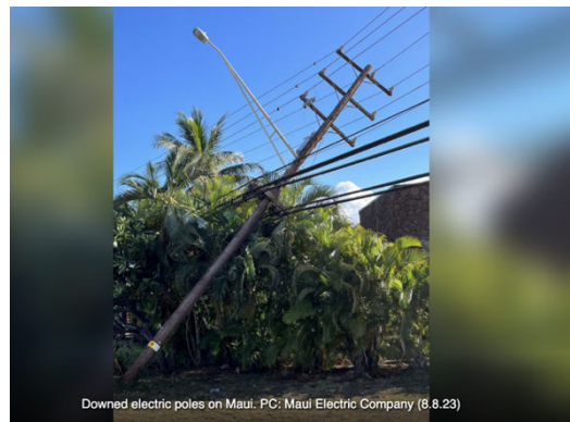
Downed electric poles on Maui. PC: Maui Electric Company (8.8.23)
