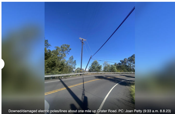
Downed/damaged electric poles/lines about one mile up Crater Road. PC: Joan Petty (9:33 a.m. 8.8.23)
