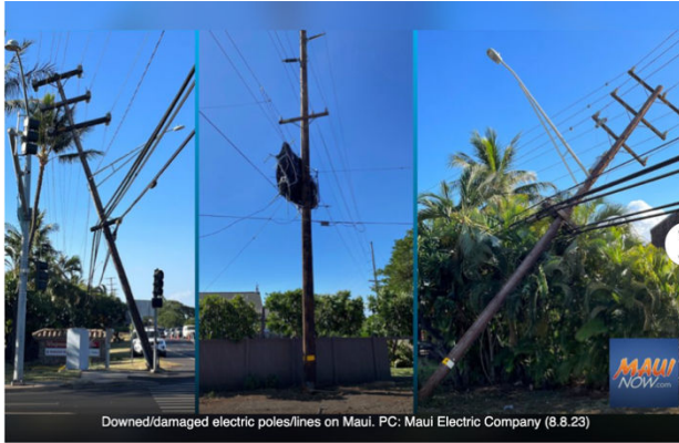
Downed/damaged electric poles/lines on Maui. PC: Maui Electric Company (8.8.23)
