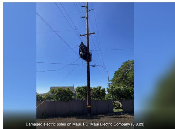
Damaged electric poles on Maui. PC: Maui Electric Company (8.8.23)
