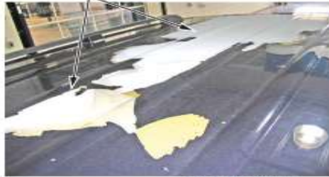
7 Example of paint peeling off in sheets from the roof.
